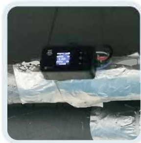
Central air-conditioning billing monitoring
