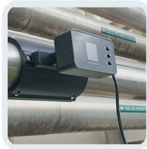
Building application flow monitoring
