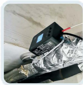
Building air conditioning cooling capacity monitoring
