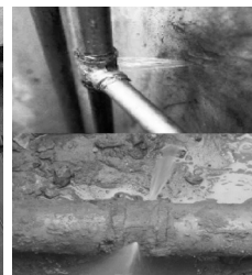
Fire Sprinkler System
